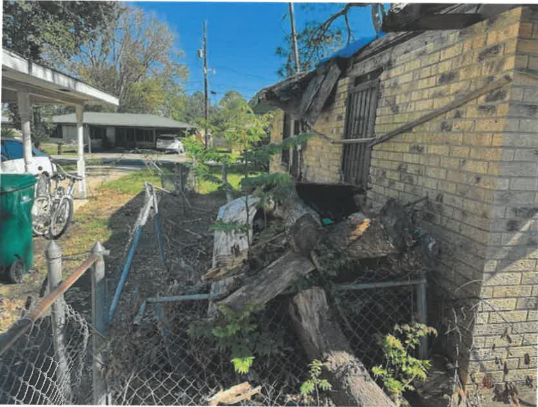
Picture taken November 15, 2024: Property has piles of downed trees causing blighting and creating habitat for pests and vermin, roof heavily damaged and falling away, open to the environment allowing moisture to enter and deteriorate interior of structure.
