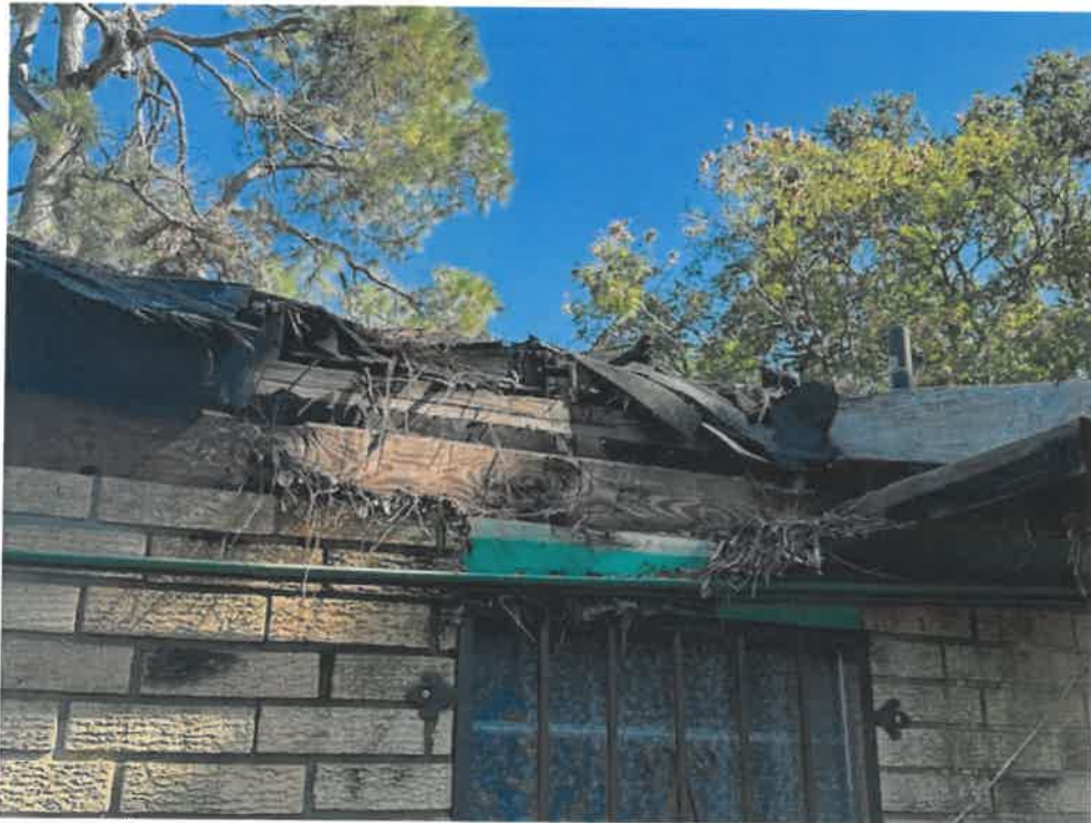
Picture taken November 15, 2024: Roof heavily damaged, open to air allowing moisture, pests and vermin to enter structure leading to further damage.
