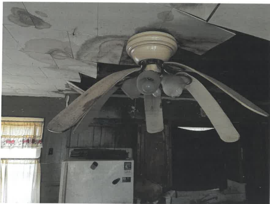
Picture taken March 27, 2025: Fan shown to be in dilapidated condition due to amount of moisture in dwelling from apparent roof damage.
