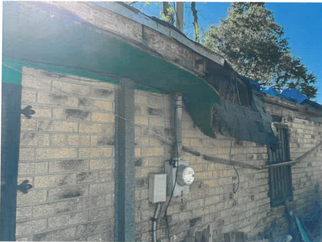
Picture taken November 15, 2024: Wiring running side of structure, roof heavily damaged and falling away, open to the environment allowing moisture to enter and deteriorate interior of structure, rubbish and debris causing blighting.
