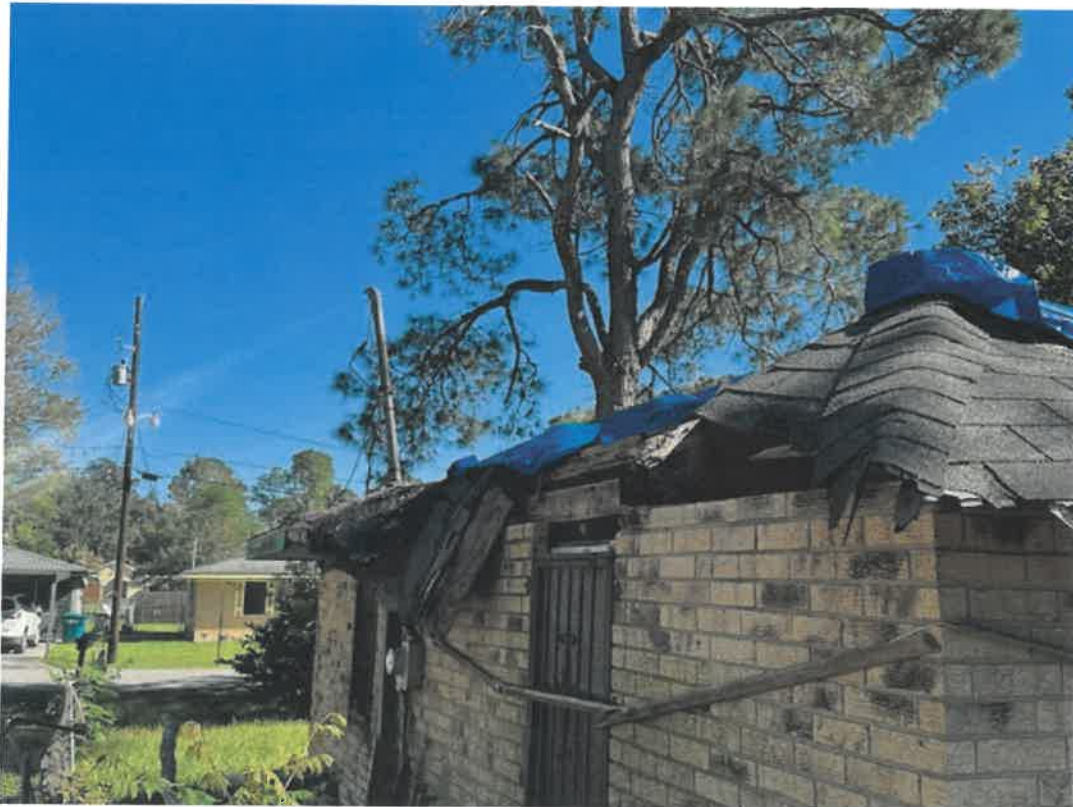
Picture taken November 15, 2024: Roof heavily damaged and falling away, open to the environment allowing moisture to enter and deteriorate interior of structure.
