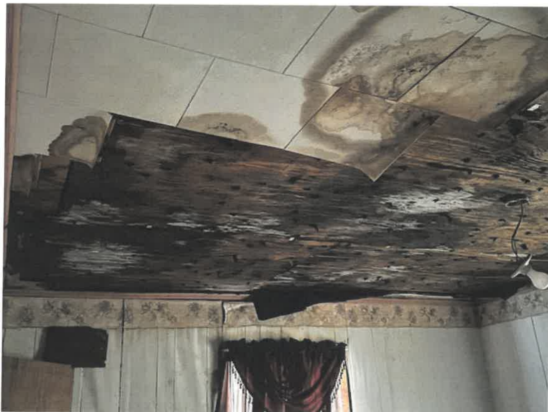
Picture taken March 27, 2025: Roof sheathing / material shown to have discoloration from water damage. This could lead to structural instability in roof system. This is in one of the bedrooms.
