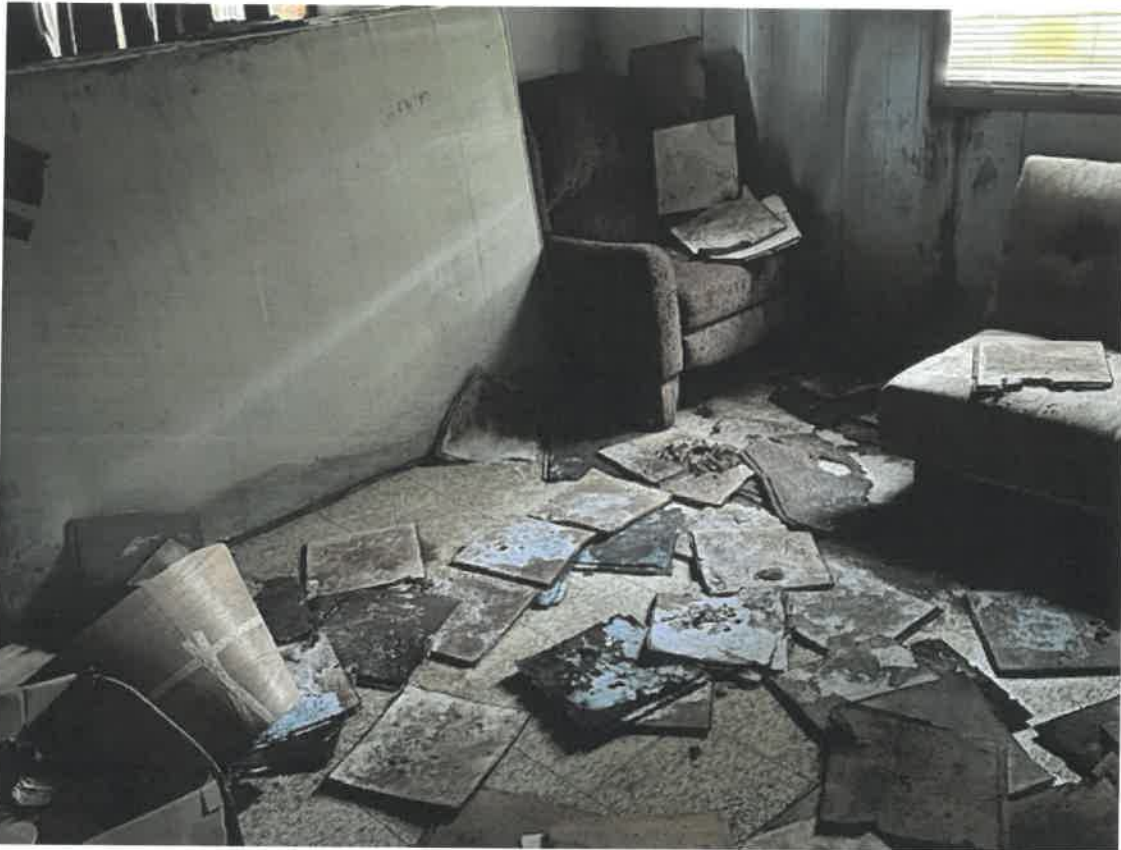
Picture taken March 27, 2025: Ceiling material shown to have fallen on ground from apparent roof damage.
