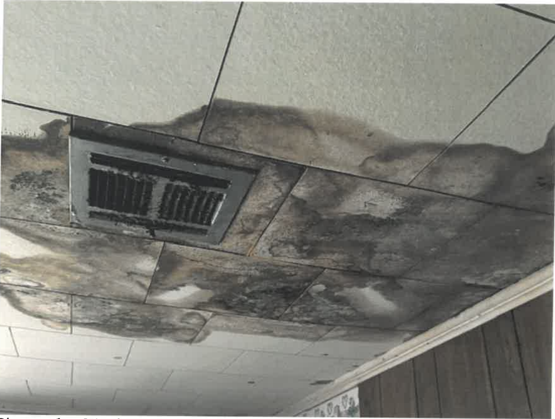
Picture taken March 27, 2025: Discoloration noted in ceiling tile appears to be cause by roof damage from fallen tree(s).
