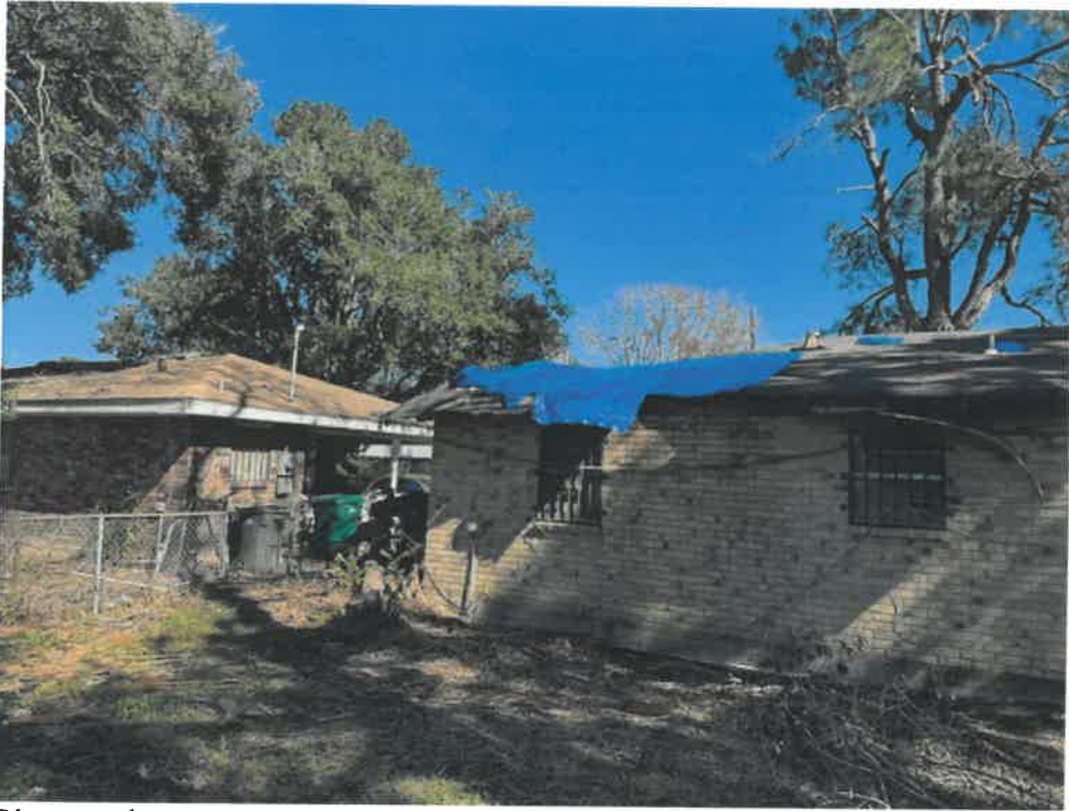
Picture taken November 15, 2024: Portions of roof covered with tarp due to tree damage to roof, large limbs remain on roof and property is overgrown with fallen limbs and foliage causing blighting and creating habitat for pests and vermin, roof damage is allowing moisture to enter structure leading to further deterioration, portions of roof rotten and falling away.
