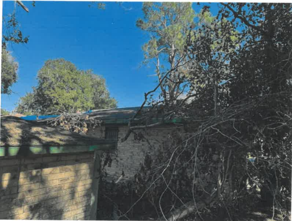
Picture taken November 15, 2024: Portions of roof covered with tarp due to tree damage to roof, large limbs remain on roof and property is overgrown with fallen limbs and foliage causing blighting and creating habitat for pests and vermin, roof damage is allowing moisture to enter structure leading to further deterioration.
