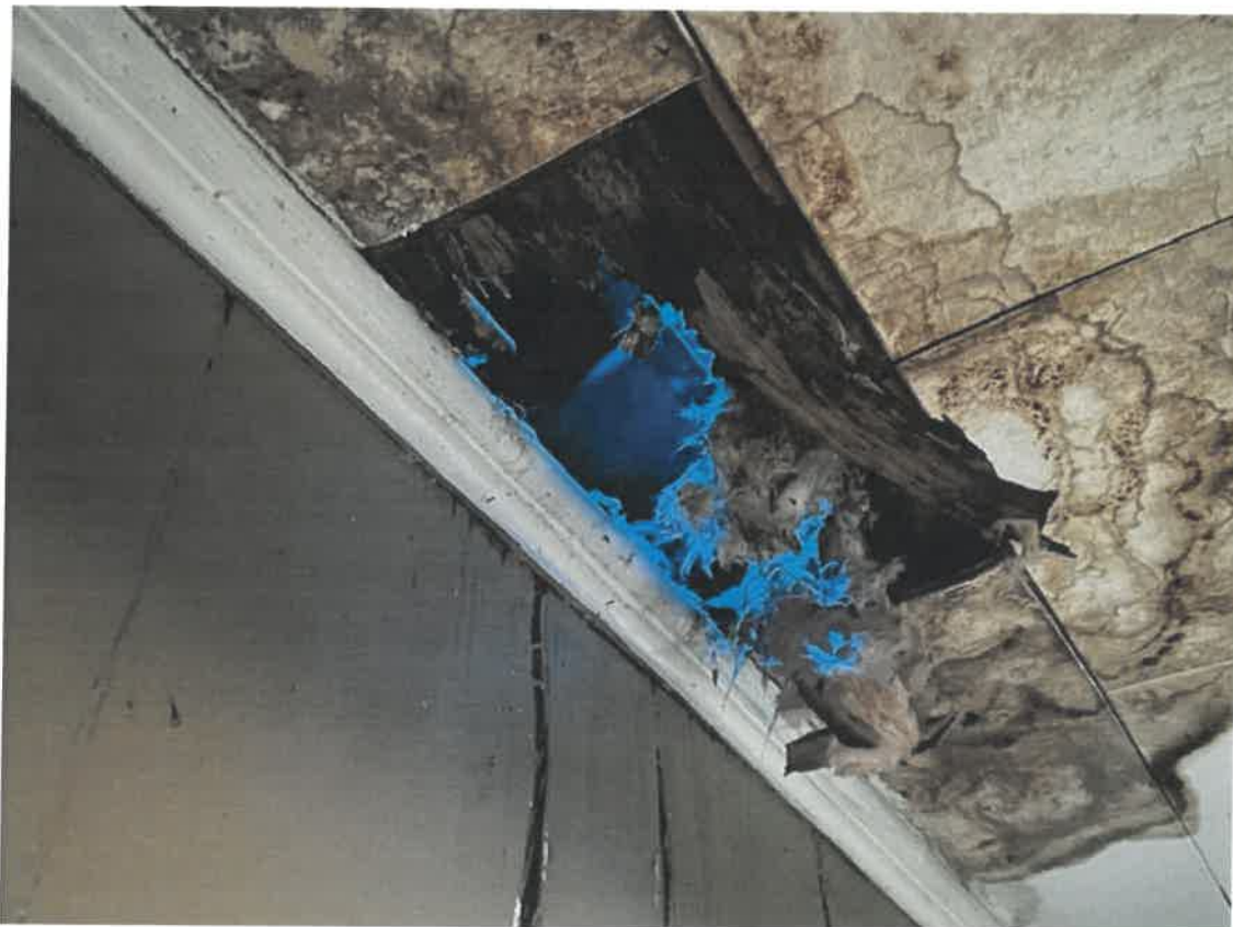
Picture taken March 27, 2025: Light showing through roof system due to damage from fallen tree.
