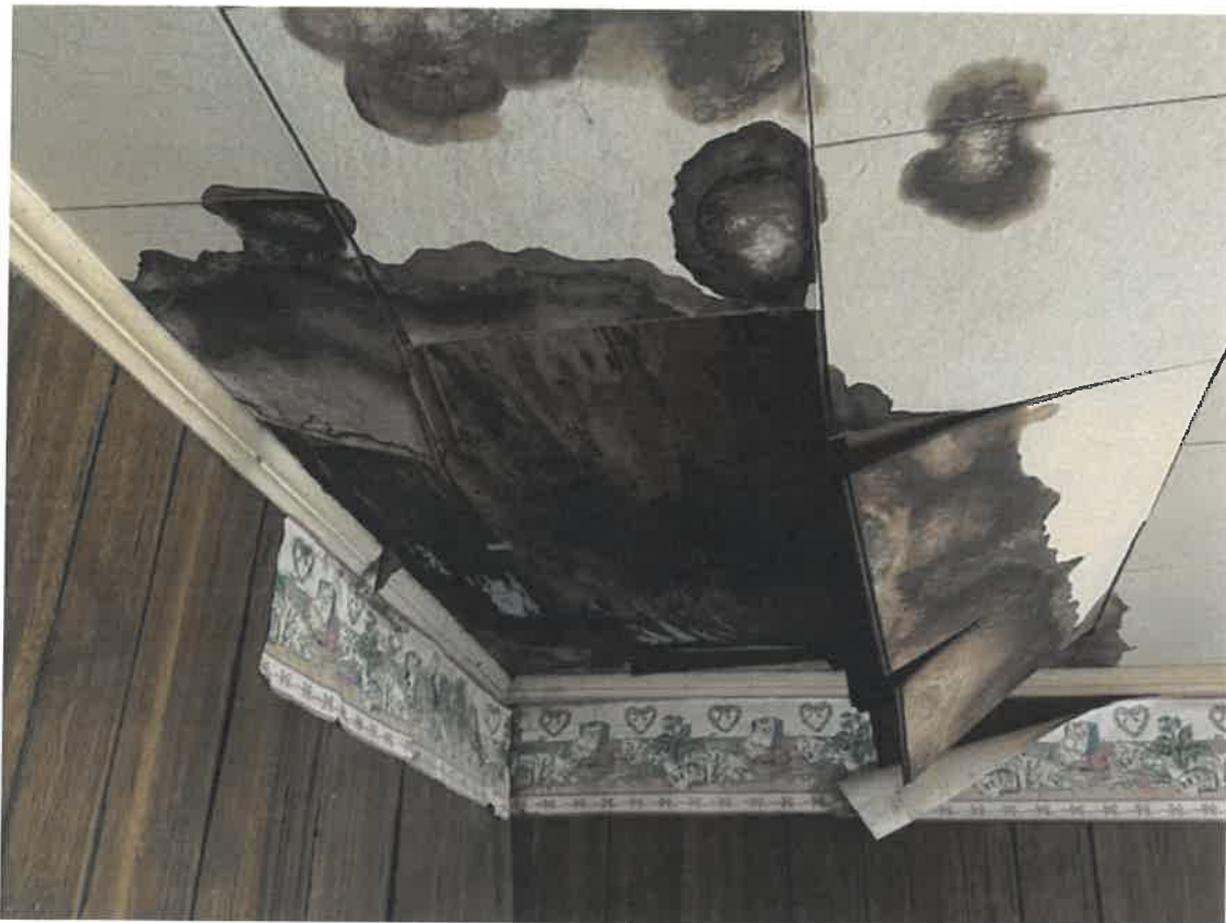
Picture taken March 27, 2025: Roof sheathing / material shown to have discoloration from water damage. This could lead to structural instability in roof system. This is in one of the bedrooms.
