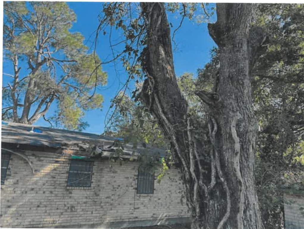
Picture taken November 15, 2024: Portions of roof covered with tarp due to tree damage to roof, large limbs remain on roof and property is overgrown with fallen limbs and foliage causing blighting and creating habitat for pests and vermin, roof damage is allowing moisture to enter structure leading to further deterioration.
