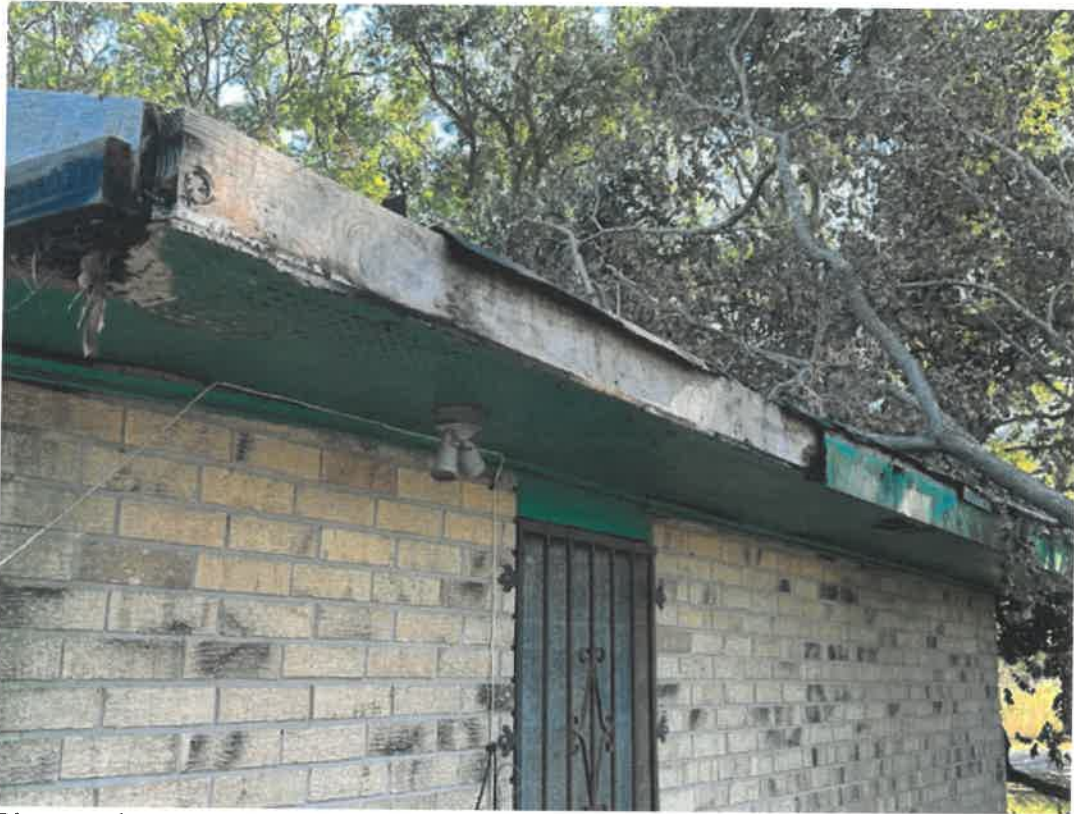
Picture taken November 15, 2024: Large limbs remain on roof and property is overgrown with fallen limbs and foliage causing blighting and creating habitat for pests and vermin, roof damage is allowing moisture to enter structure leading to further deterioration, portions of roof rotten and falling away.
