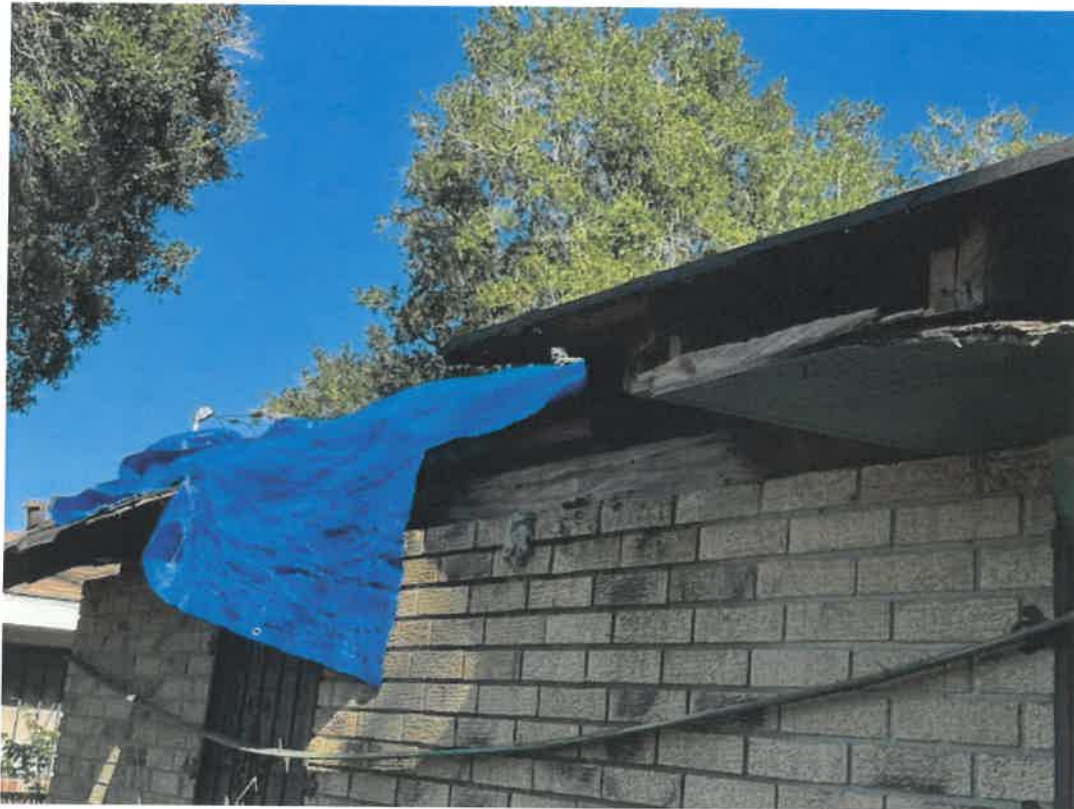
Picture taken November 15, 2024: Roof heavily damaged, open to air allowing moisture, pests and vermin to enter structure leading to further damage.
