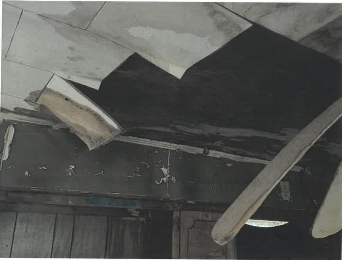
Picture taken March 27, 2025: Roof sheathing / material shown to have discoloration from water damage. This could lead to structural instability in roof system. (Kitchen)
