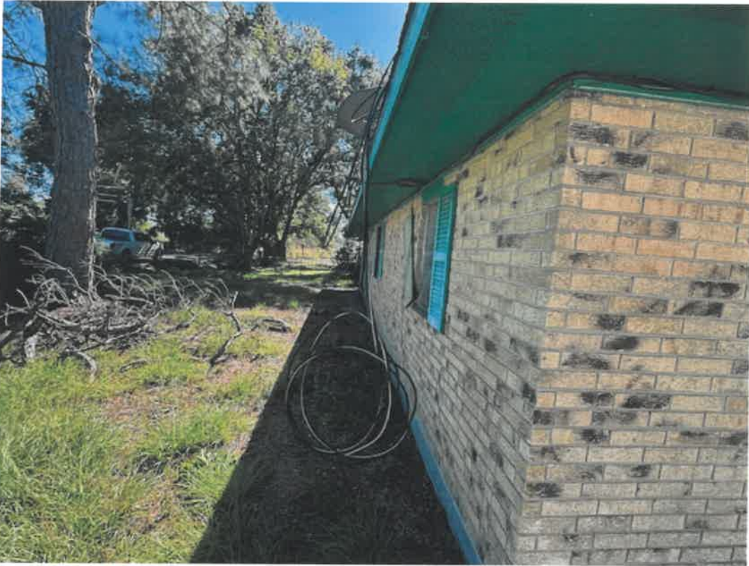
Picture taken November 15, 2024: Overhead power line on ground.
