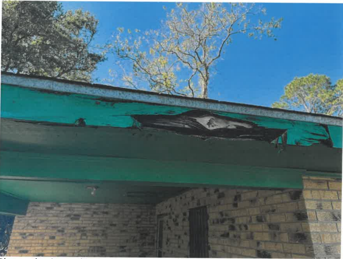
Picture taken November 15, 2024: Portions of roof boxing and fascia rotten and falling away.
