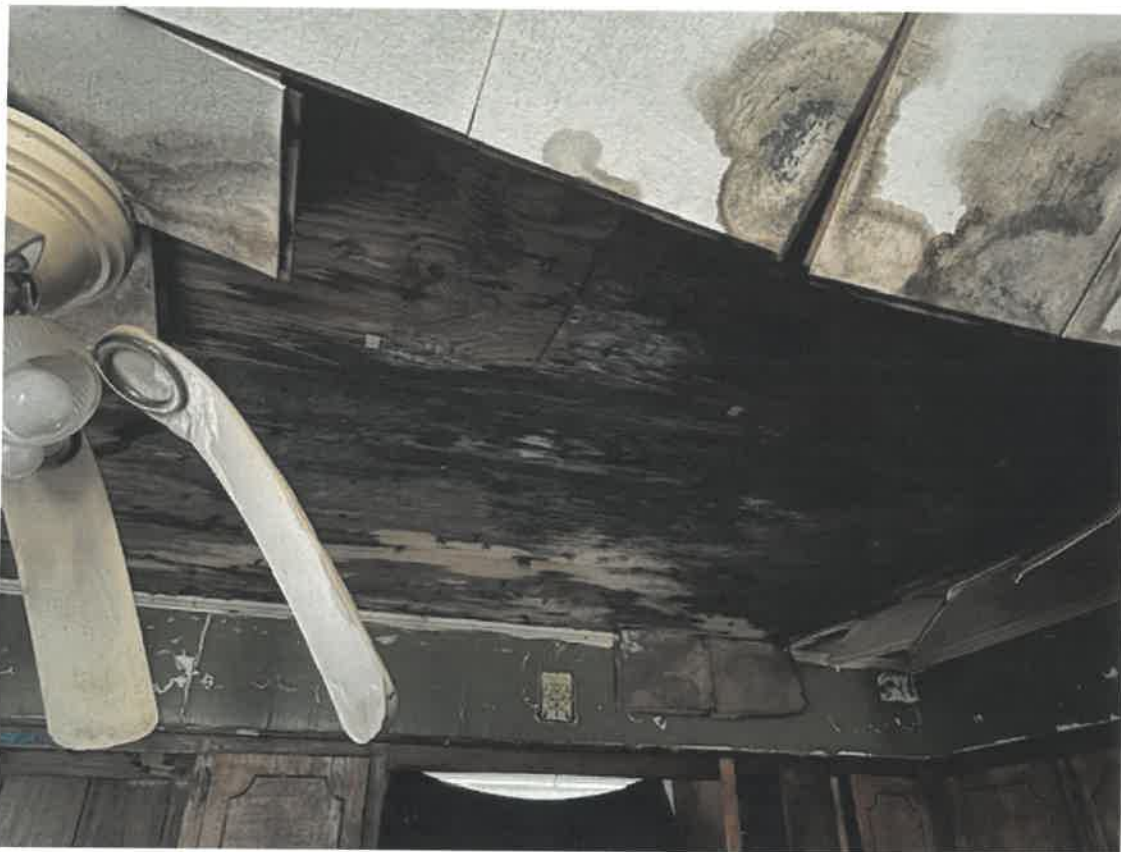
Picture taken March 27, 2025: Roof sheathing / material shown to have discoloration from water damage. This could lead to structural instability in roof system. (Kitchen)
